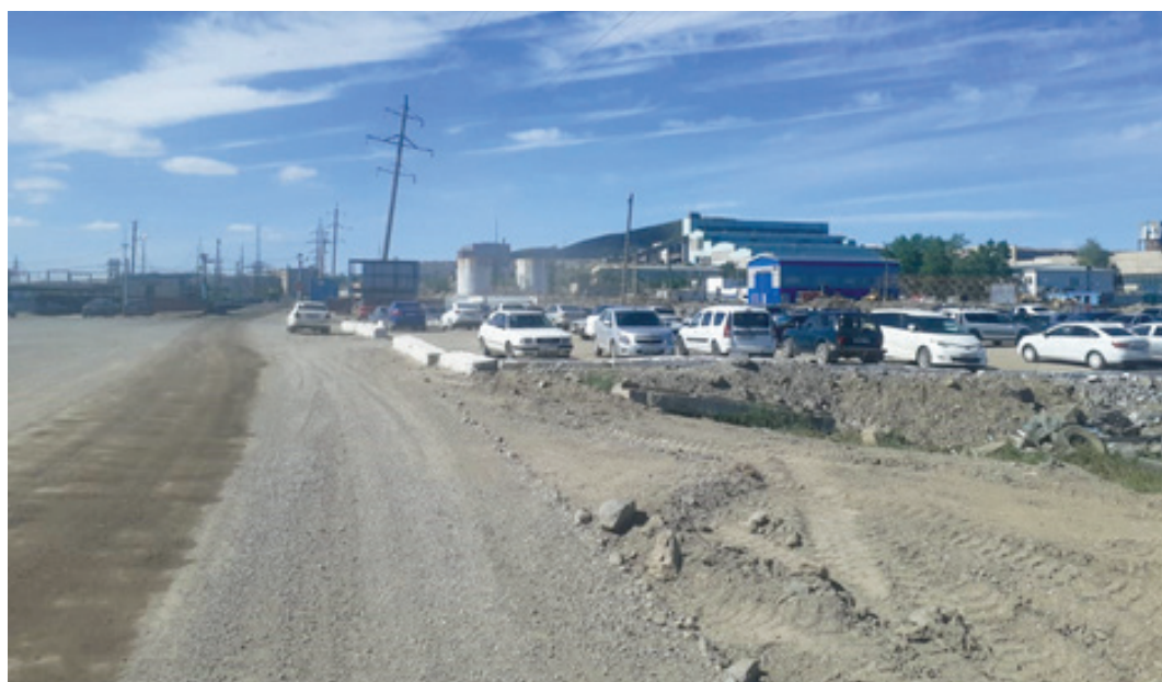
Figure 3. Karagaily Mining and Processing Plant of “Karagandatsvetmet” PA, a branch of Kazakhmys Corporation LLP (photo by the author)
